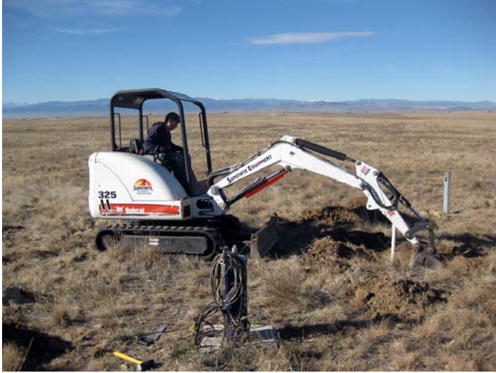
Photo 1 (below): The soil and overburden, adjacent to monitoring wells to be abandoned in Section 9, T9N, R67W, were excavated. Well IS-009-Tc is shown in this photo.
