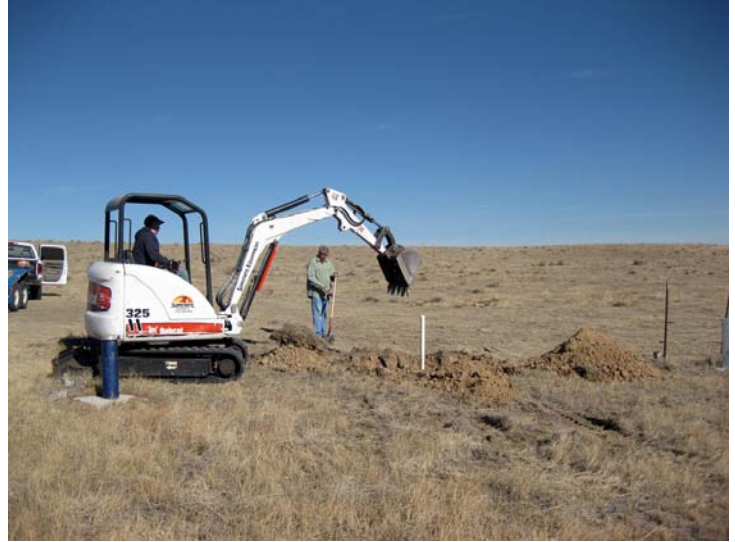
Photo 2 (above): Excavation of soils and overburden, to a depth of approximately 30 inches, was performed adjacent to monitoring wells to be abandoned in Section 33, T10N, R67W. . Note topsoil stockpile. Well IS-003-Tc is shown in this photo.
