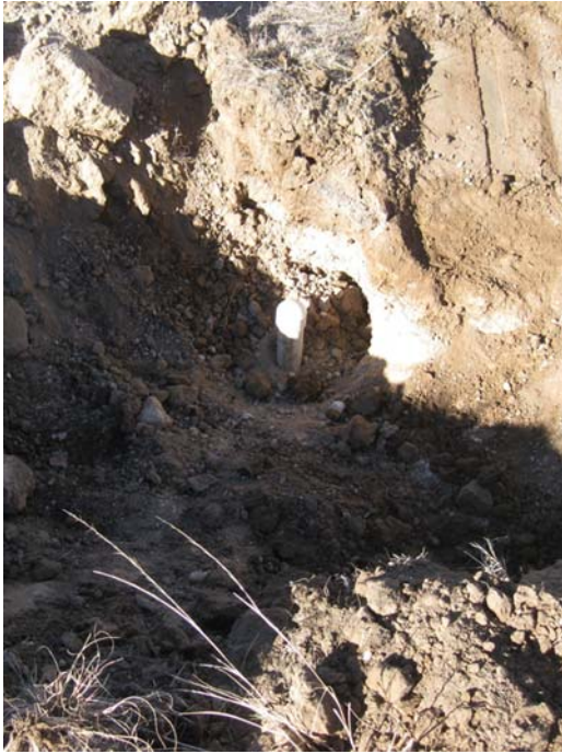
Photo 5 (above): After sand and bentonite was placed into the casing, a PVC cap was glued to the top of the casing to prevent entry of surface fluids into the casing.
